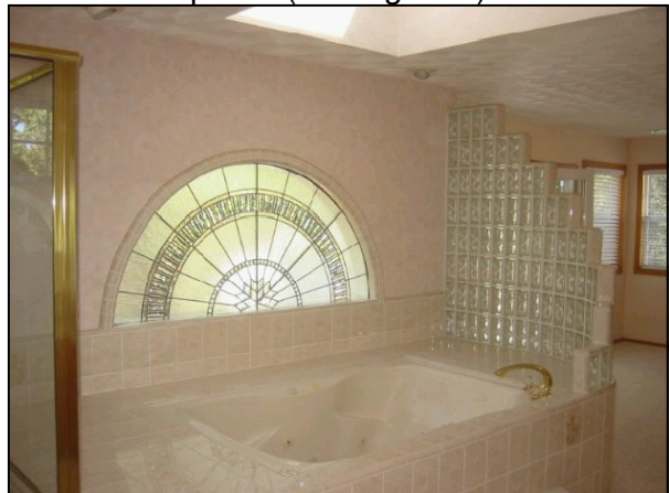
Figure 6 – Shower and Tub Enclosures In this example, the shower enclosure at the left contained tempered safety glass, and the glass blocks at the end of the tub are exempt. The leaded glass next to the tub is not allowed; any windows in that area must be safety glass.
