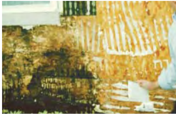
Figure 10. This wall shows characteristic damage from leaks at the window frame joints. Good flashings and a drainage plane would have saved the structure.
