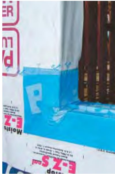
Figure 8. Sealing window flanges to the housewrap (far left) is a common practice, but it does not protect against the predictable leakage within the window assembly itself. Only a pan flashing that dumps on top of the drainage plane will effectively keep water out of the wall. Peel-and-stick membrane applied over the top of the building paper and wrapping the sides and bottom of the rough opening (left) accomplishes the task. A preformed metal pan flashing with soldered joints (below) also works. The author highly recommends Tyvek FlexWrap for pan flashings, whether the drainage plane is housewrap or rigid foam (below left).
