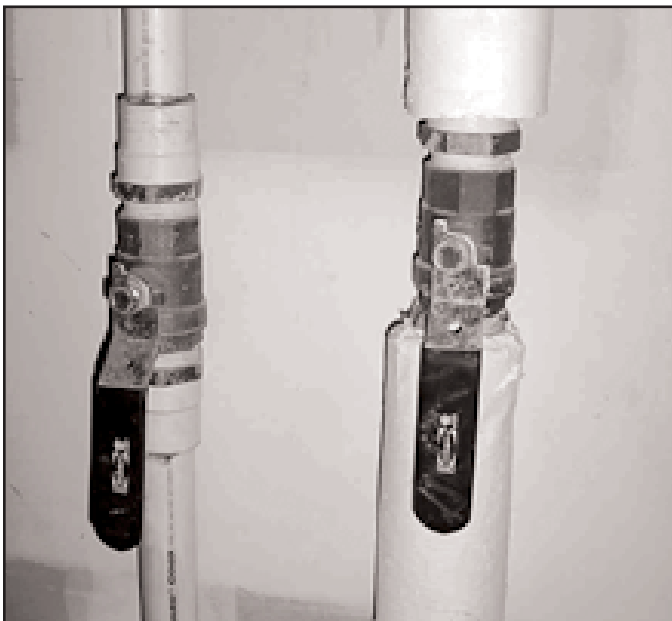
Valves installed with FlowGuard Gold® pipe.
