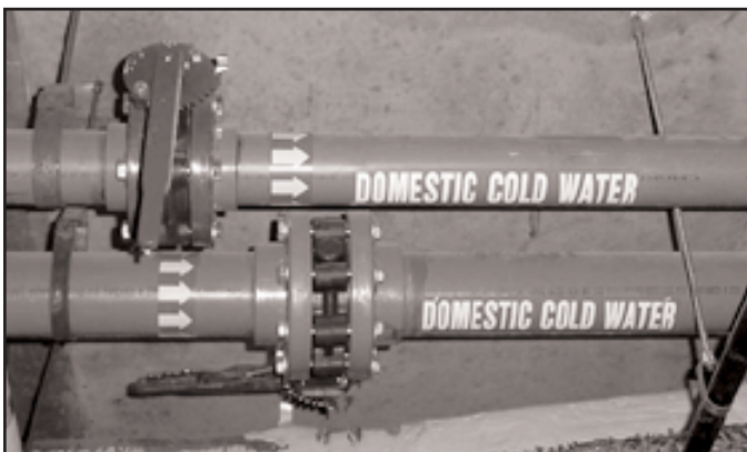
Butterfly valves installed with Corzan® pipe.
