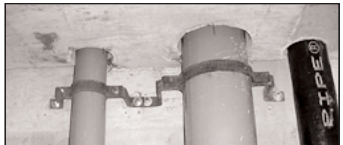
Typical riser supports using Corzan® pipe.
