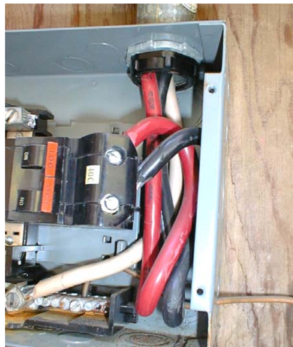
Figure 1 – Insufficient wire bending space
